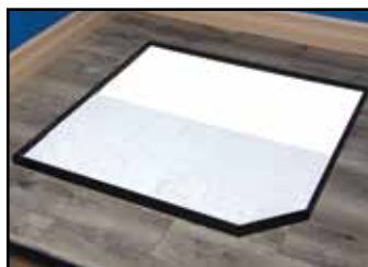
10. Lay in the Cement Board triangle piece and (1) 12" x 36" Cement Board rectangle piece.
